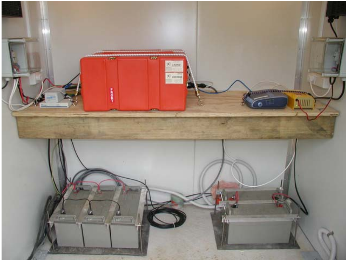
Figure 4. A photograph of the inside of a NZNSN equipment hut showing the orange Quanterra Q4120 to the left and the VSAT indoor unit to the right on the bench. The digitiser and VSAT communications equipment have separate power supplies with backup batteries on the floor of the hut. This site also records the data from a CGPS station (using a Trimble NetRS) via a Freewave Ethernet Bridge radio to the left of the Quanterra.
